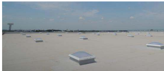
Milšped, Krnješevci - svetlosne kupole
